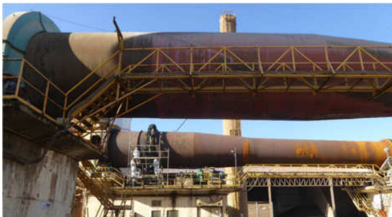
Figure 1 – Partial view of the kiln that suffered the failures, in the background. In the foreground, another kiln decommissioned since 2011.
