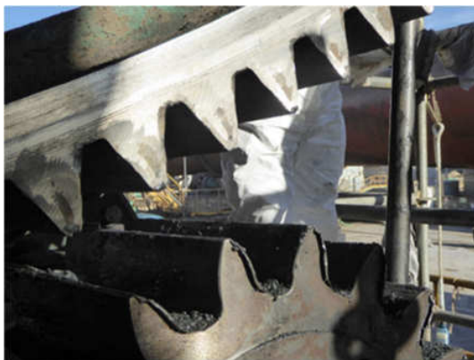
Figure 4 - Toothed crown and pinion. The teeth of the pinion show plastic flow of material outside the teeth width; at a lower scale this also existed in the toothed crown but that plastically deformed material was removed during the present stoppage.
